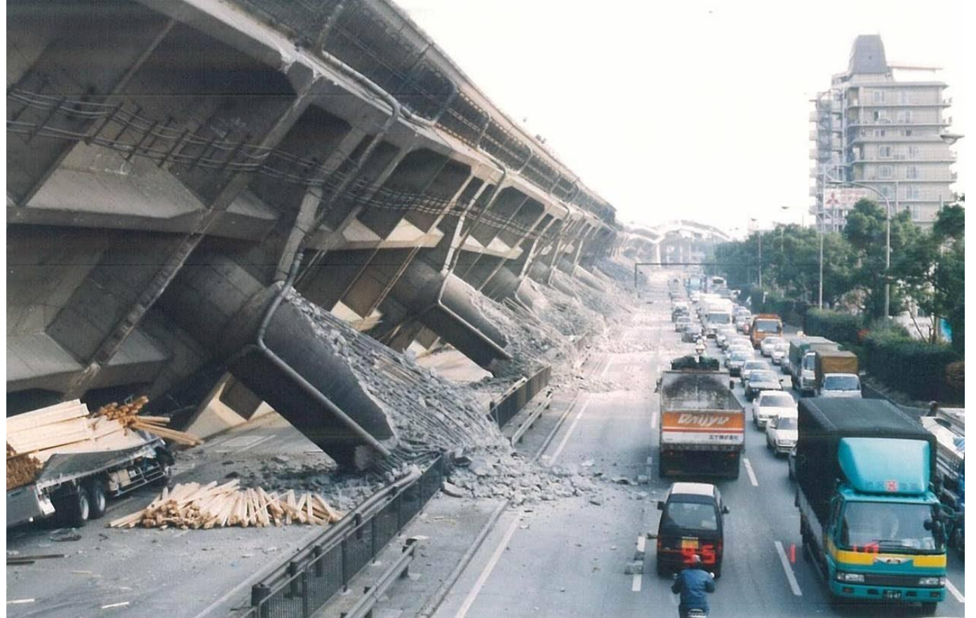
Collapsed Hanshin Expressway. Kobe Earthquake. Japan, 1995.
